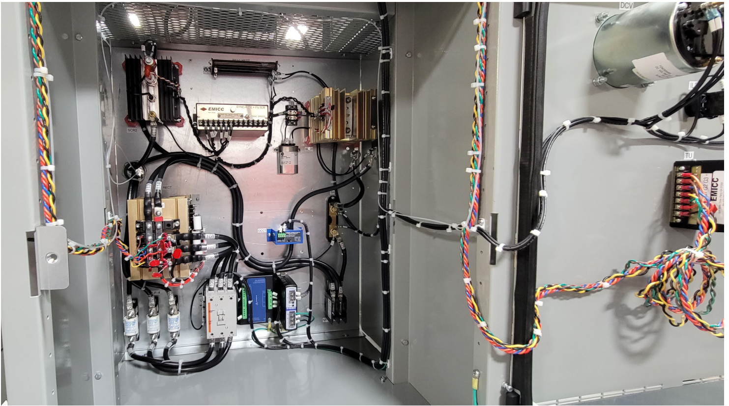
Synchrostatic field control complete with Synchronex static exciter.
